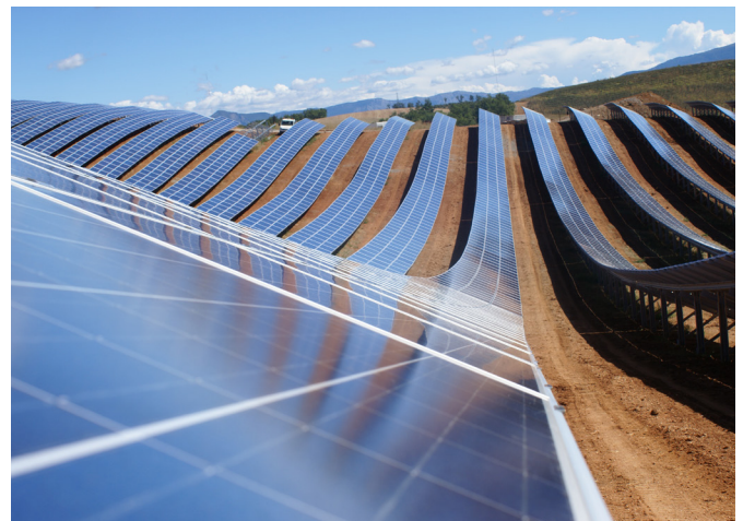
Doric Solar Provence
